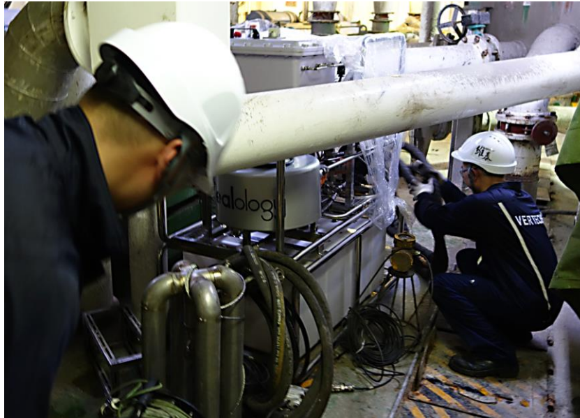
Fig1. Vertechs REALology is deployed in a confined & limited space on the drilling platform.
